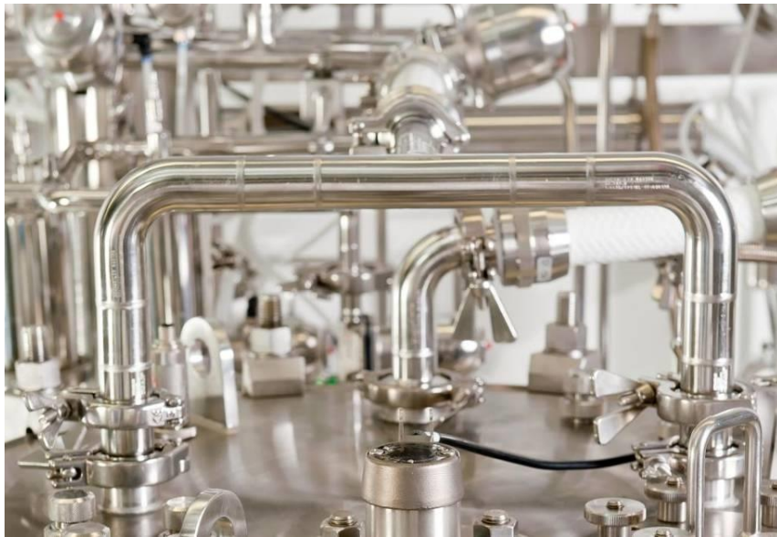
Spray ball piping (200L)
